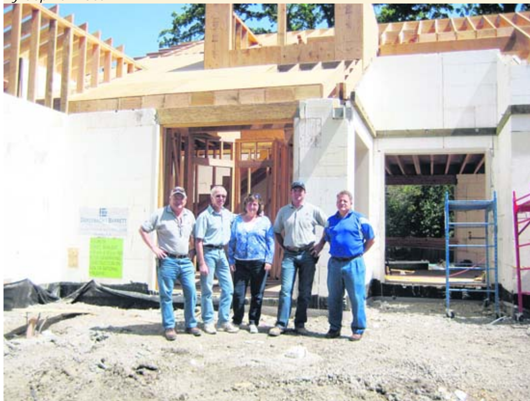
Home built with ICFs in Lafayette; (left to right) Marty Diefenbach, Gary and Rica LaVerda (property owners), Jeff Barrett and John Campaglia (project manager with Diefenbach and Barrett) Photo Sophie Braccini
