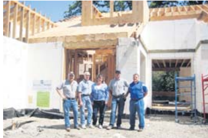
Home built with ICFs in Lafayette; (left to right) Marty Diefenbach, Gary and Rica LaVerda (property owners), Jeff Barrett and John Campaglia (project manager with Diefenbach and Barrett) Photo Sophie Braccini
