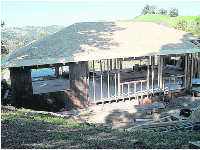
Current view of Ruth Court house, construction should be completed in March.
