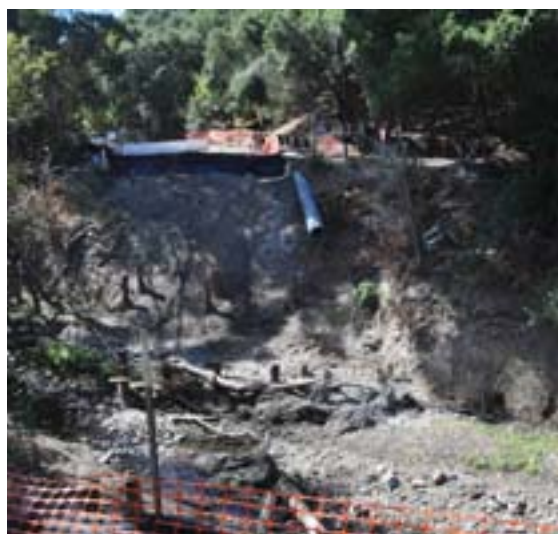
The bridge is gone Photo Andy Scheck
