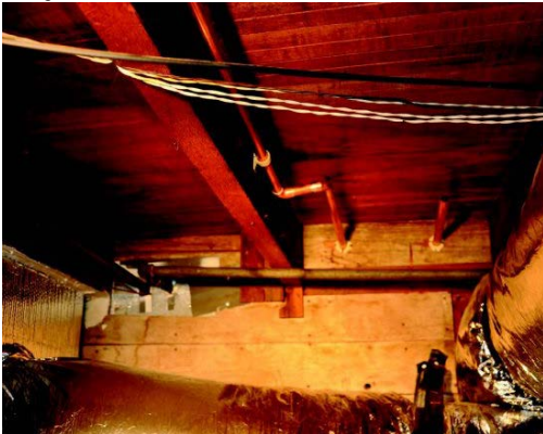
New copper piping on top and old pipes below. Photos Andy Scheck
