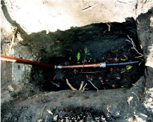
The new copper pipe is connected to the water main outside the house.
