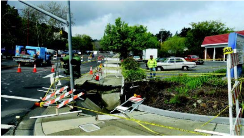
This sinkhole developed in March 2016 Photo provided
