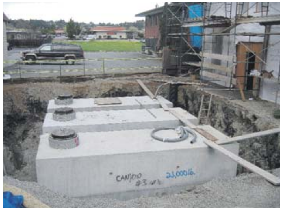
Concrete tanks were buried by "The Barn" at the time of its renovation.
