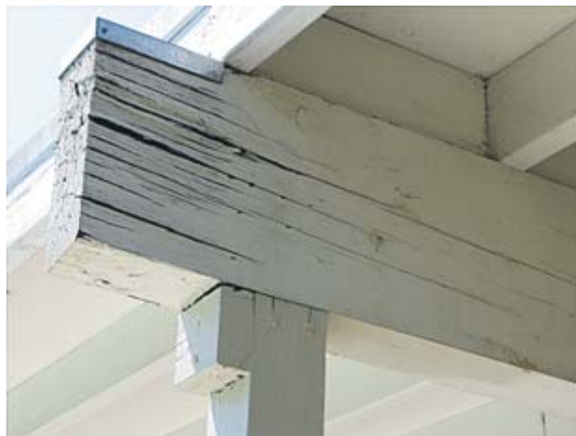
Dry rot on a roof beam
