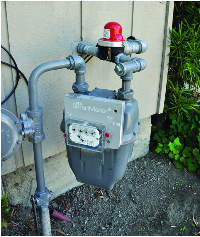
Gas meter with seismic valve
