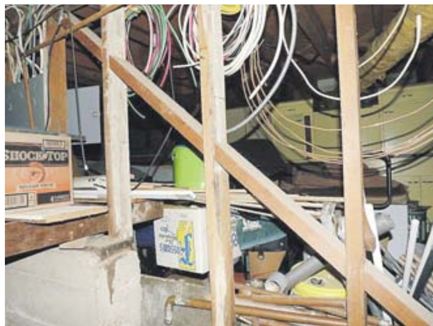
An example of cut-in braces on a cripple wall that does not offer seismic bracing
