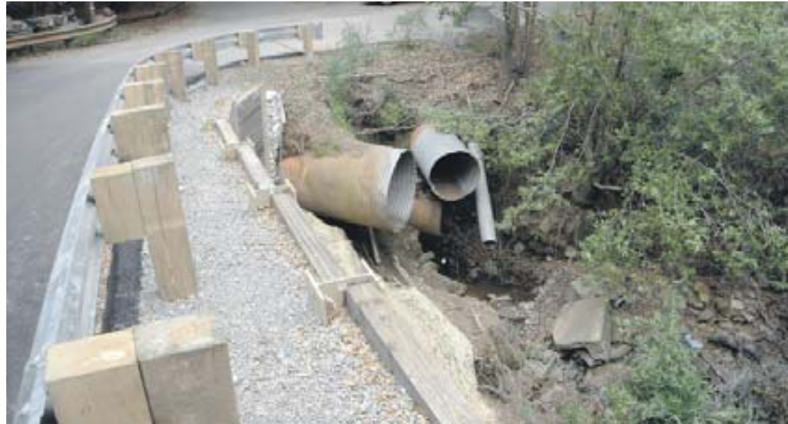
Repairs to an El Toyonal roadside drainage ditch have been added to the City of Orinda's updated Capital Improvement Plan for 2012-2013. Note the aging corrugated metal pipe (CMP). Estimated price tag: $30,000. Photo provided
