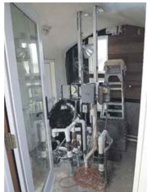
The Walters' pump house Photo Cathy Dausman
