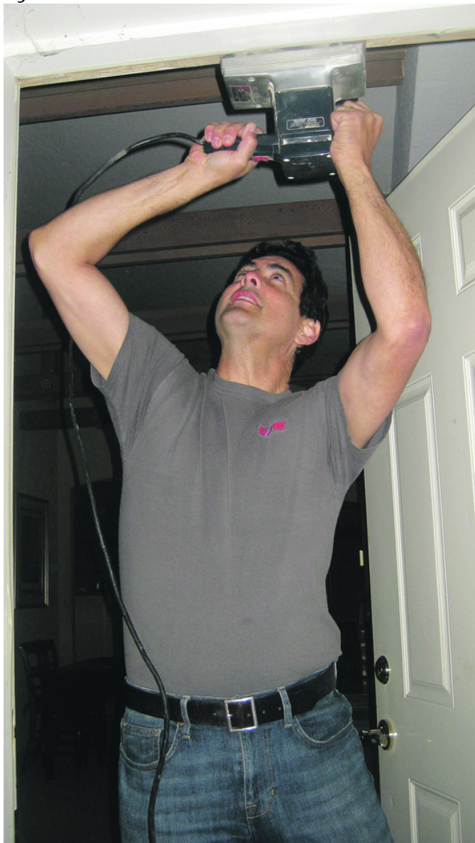
Mark Shaw works on a sticking interior door at his home in Orinda. Photos Chris Lavin
