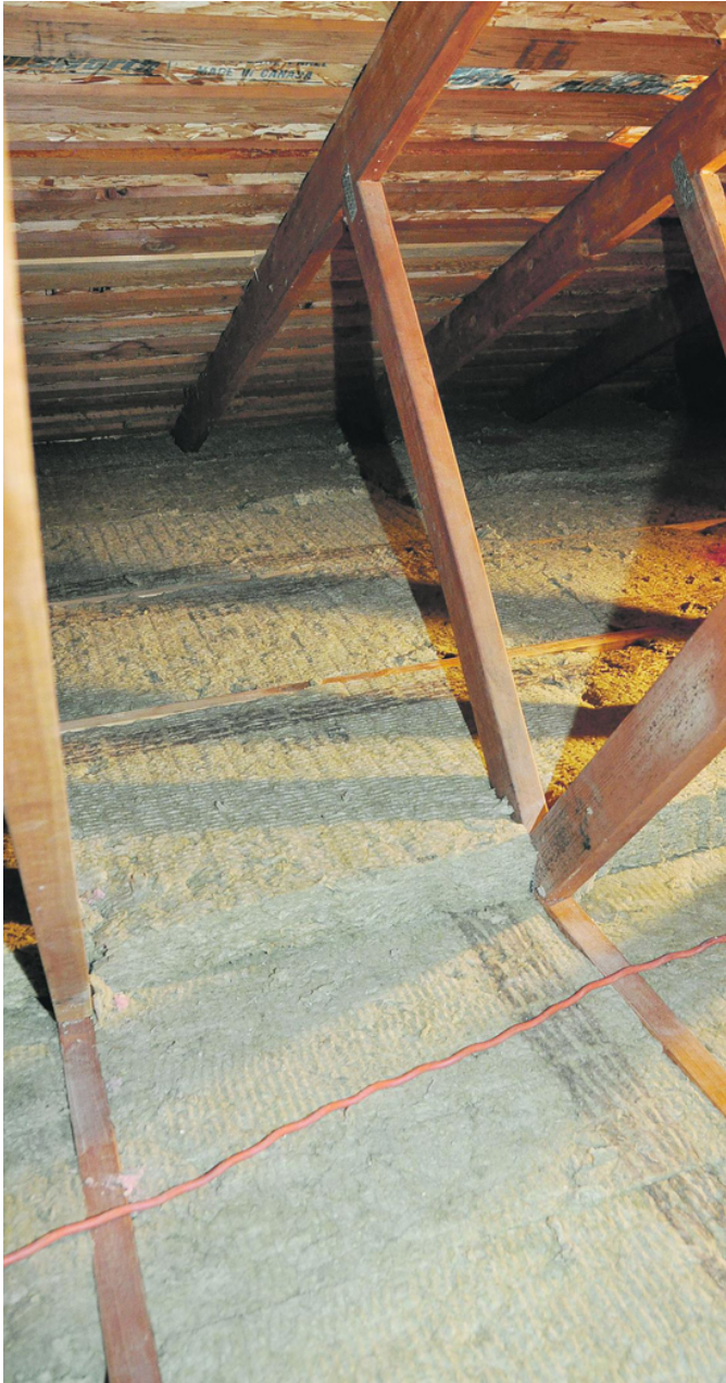
Two perpendicular layers of stone wool insulation batts were easy to install in this Moraga home. Photo Andy Scheck
