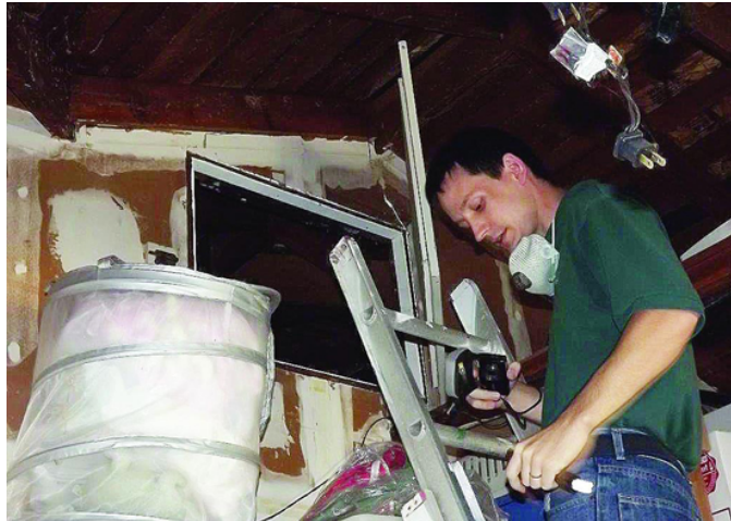
Kyle Bosworth of Eco Performance Builders inspects the Penneys' home. Photo Cathy Dausman
