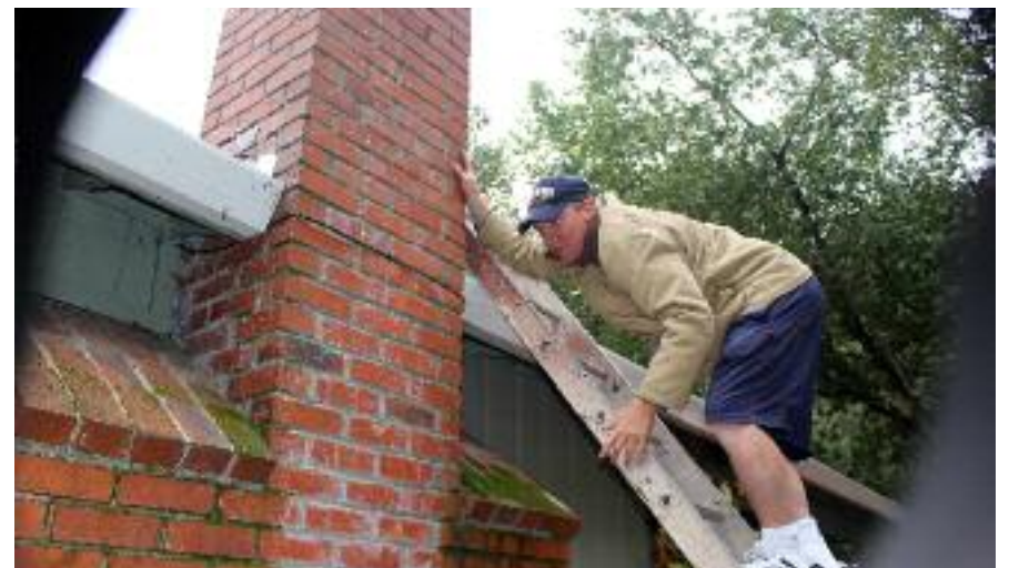
Dylan Llewellyn checks out a neighbor's brick chimney for rot.
