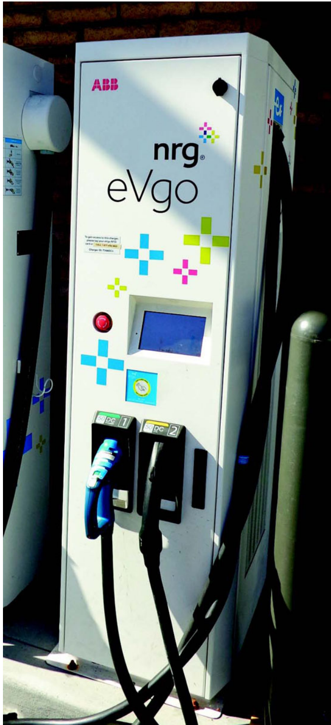
EVgo pump at Whole Foods Market in Lafayette. Photo C. Tyson
