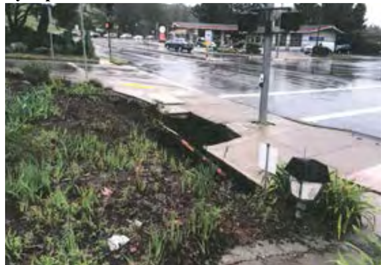
Sunday, March 13: The initial emergence of sinkhole.
