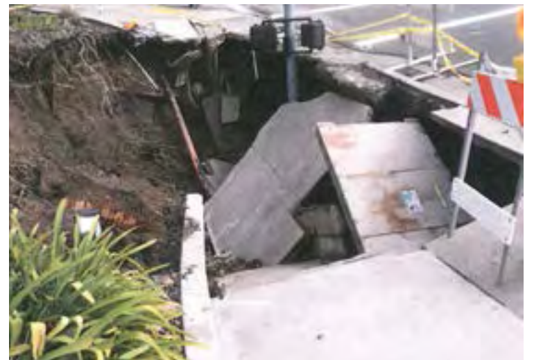
Monday, March 14: A traffic signal pole, a PG&E electrical switch vault and portions of the sidewalk collapsed into the sinkhole. Photos provided
