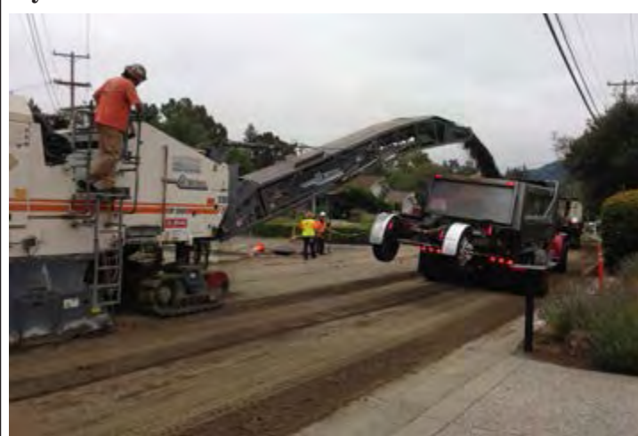
Repaving on Ivy Drive in Orinda is just one local roads improvement project. Photo Victor Ryerson
