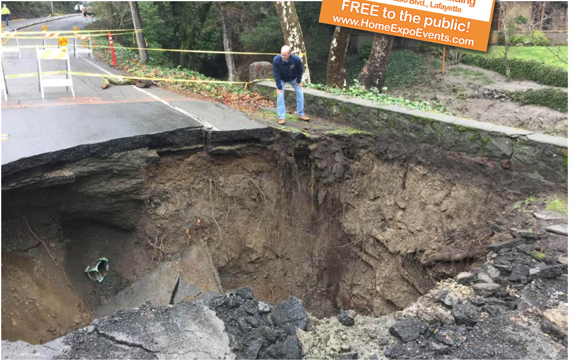
State Senator and Orinda resident Steve Glazer inspects the sinkhole on Miner Road.
