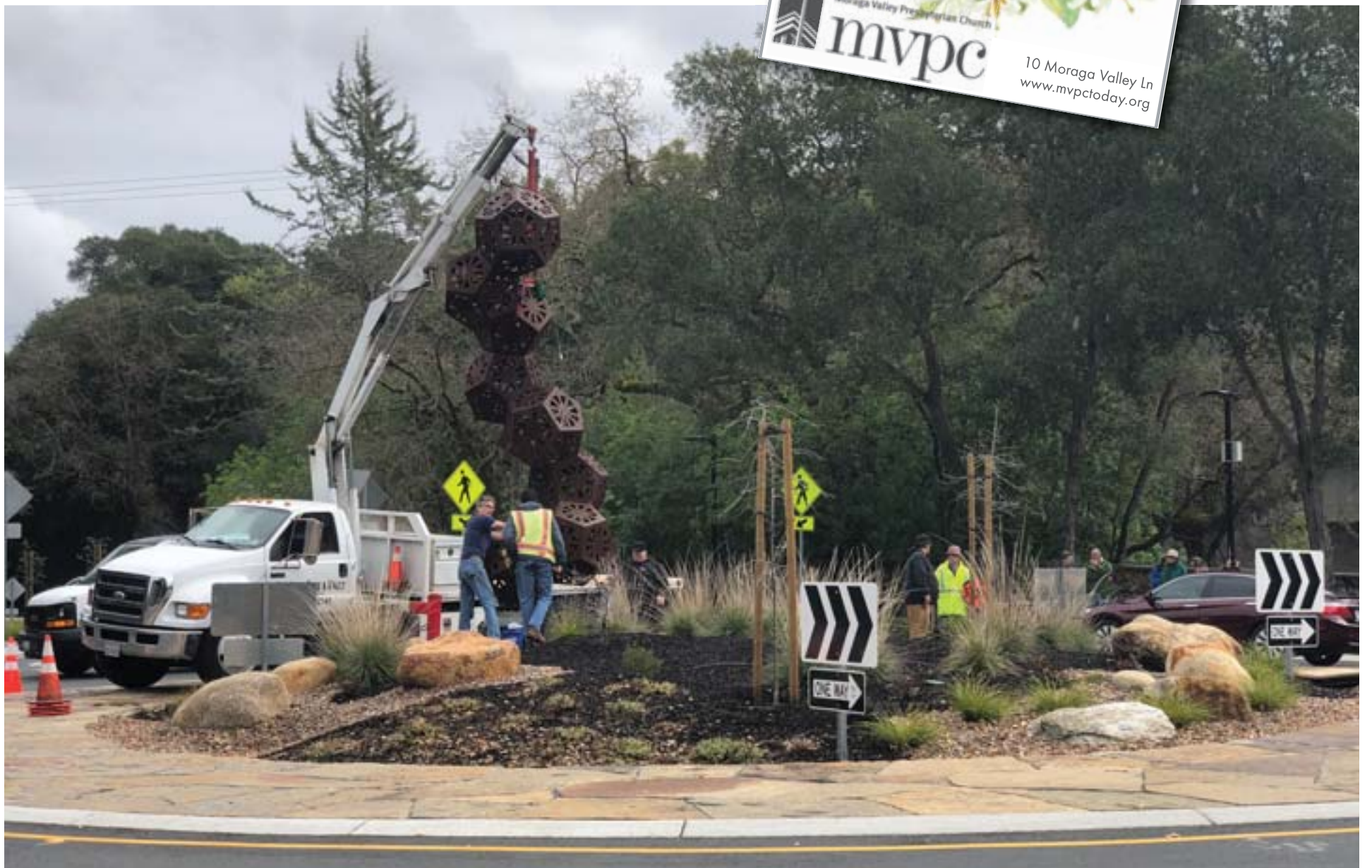
Local artist David Mudgett, on left, works to install "Resolve" with city staff on the new roundabout March 13.
