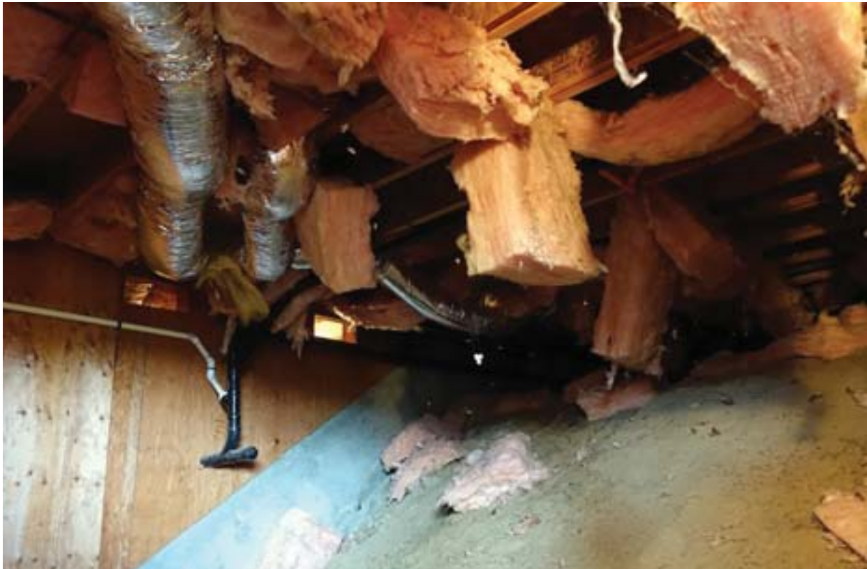
Rats may disturb the insulation from between the floor joists. After the slab cures insulation must be re-installed.
