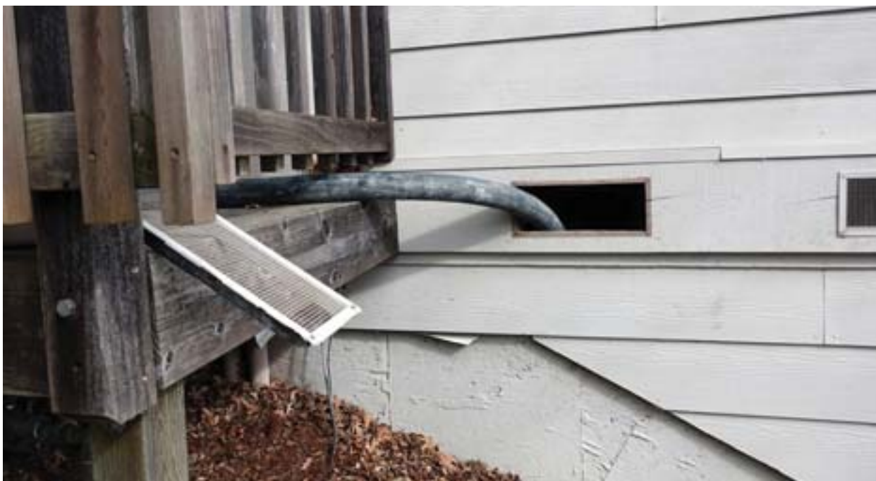
Concrete is delivered into the crawl space via the easiest route – in this case, a vent opening.
