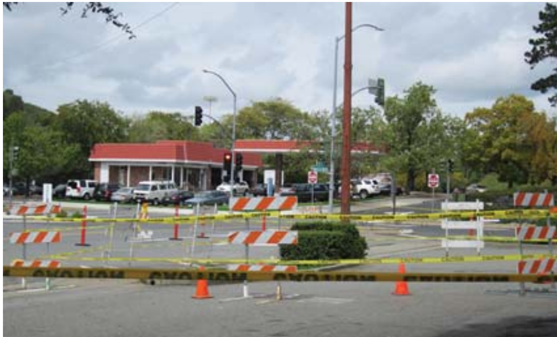
Cordoned off area of sinkhole
