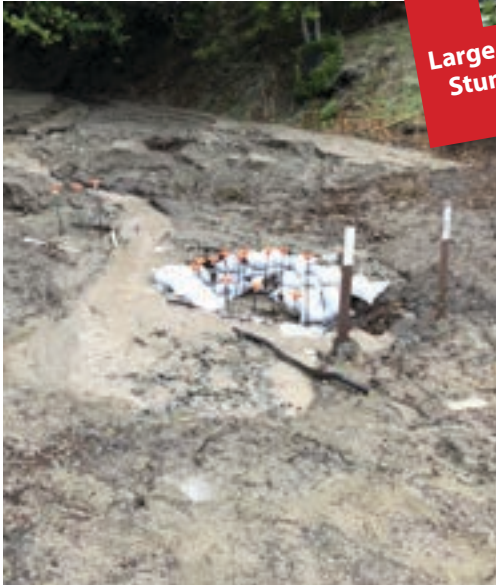
Buried storm drain inlet flooded roadway at Bollinger Canyon Road
