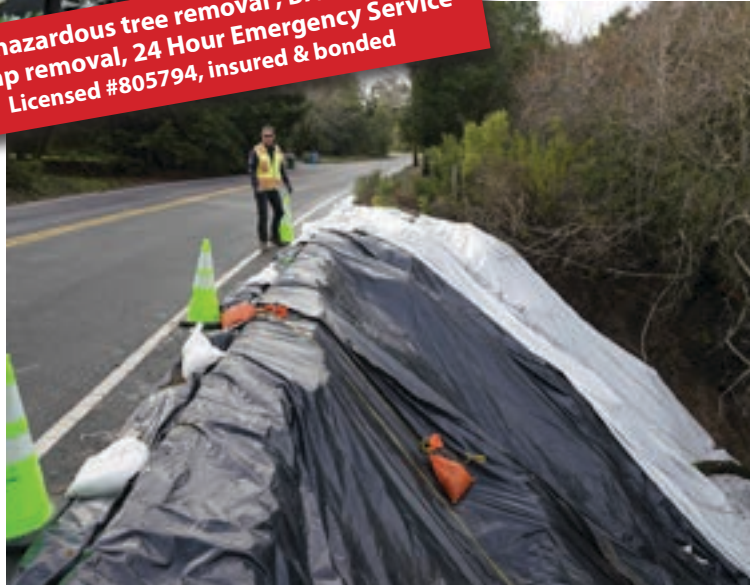
Public Works Director Mike Moran inspects segment of storm damaged shoulder of St Mary's Road near Driftwood Drive
